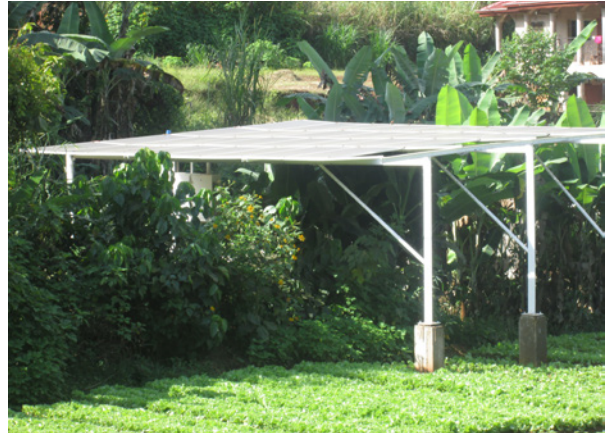
Picture 19. PB funded solar panel installation for drinking water pumping and distribution, Nyom neighbourhood © Yaoundé Commune 1
