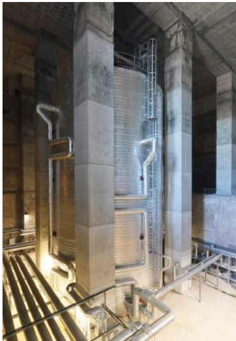
□ The Firstly Built Energy Box in Hamburg
